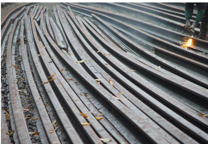
Hand Cutting Scrap Rail Strings Removed from the Tunnel Prior to Sale Photo by Phil Corder
