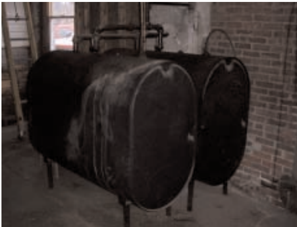
Before - Two unlabeled tanks
